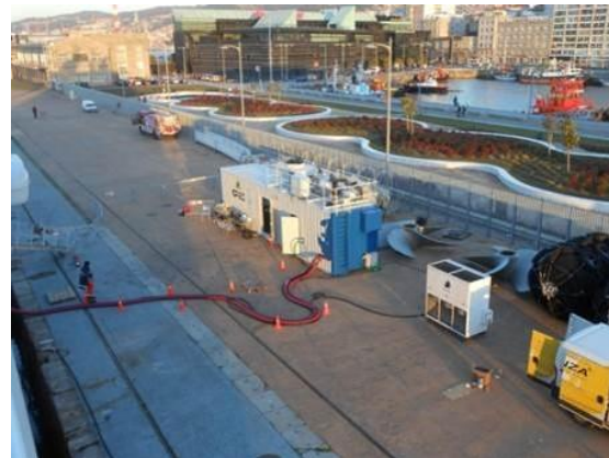
Polygeneration clusterizable containerized system that supplies electrical and thermal energy to the ships.
